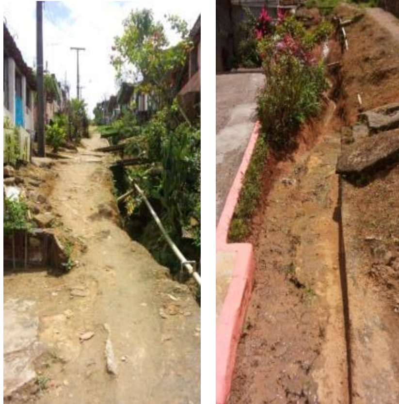
Figuras 40 (1, 2) - Vala irregular
