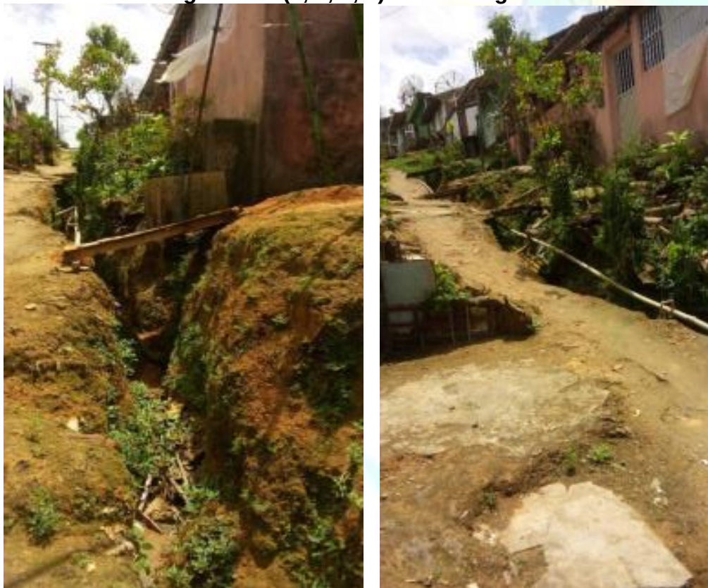
Figuras 39 (1, 2, 3, 4) - Vala irregular
